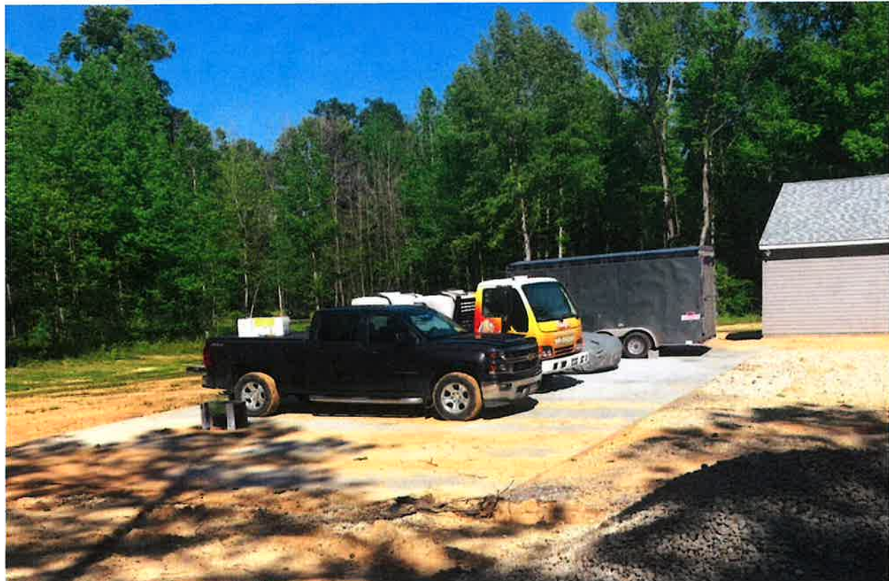
View of concrete pad (proposed building location). West side of house visible at right.
