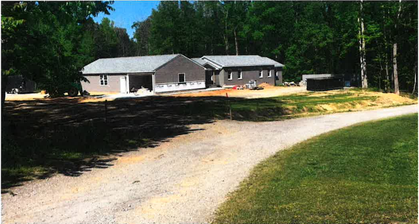
View of Southwest of house from Silvercrest Lane roadway. Black trailer parked on concrete pad (proposed building location) to left of house. Shipping containers and temporary dumpster at right of house.
