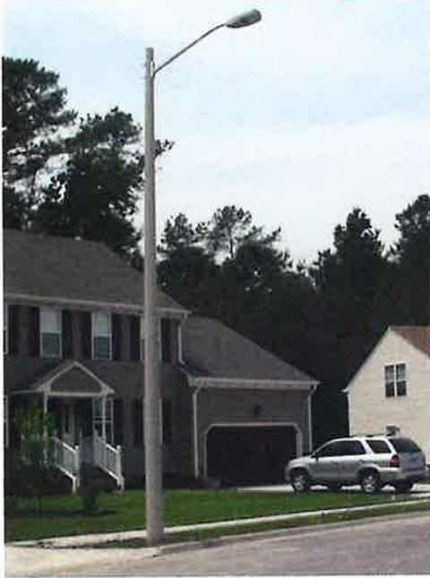
Enclosed on concrete or composite pole
